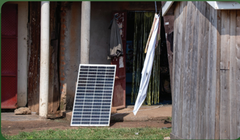
Solar energy panel system in Kijumba ,Hoima district
