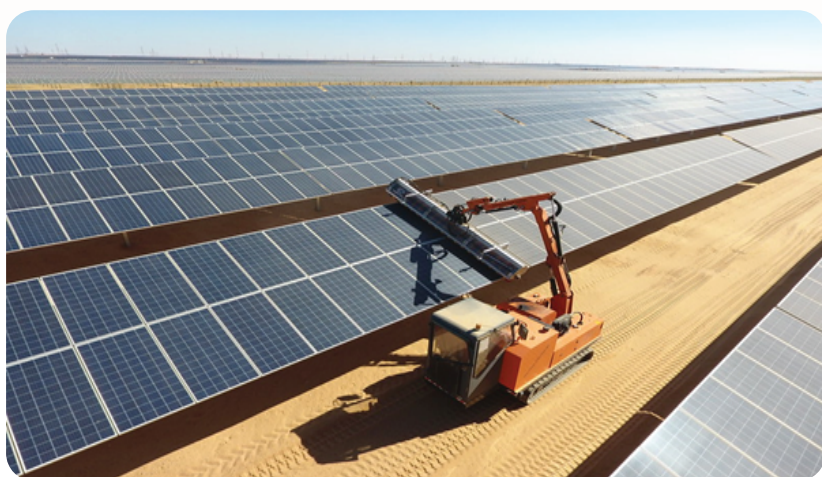
A photo of the Egypt - Benban Solar Park, Solar Photovoltaic Power Project under the Egyptian Feed-in-Tariff Program Round 2 - Alcazar Energy Egypt Solar 1
